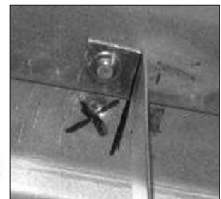
M034 fastener used to hang HVAC Duct Strap
