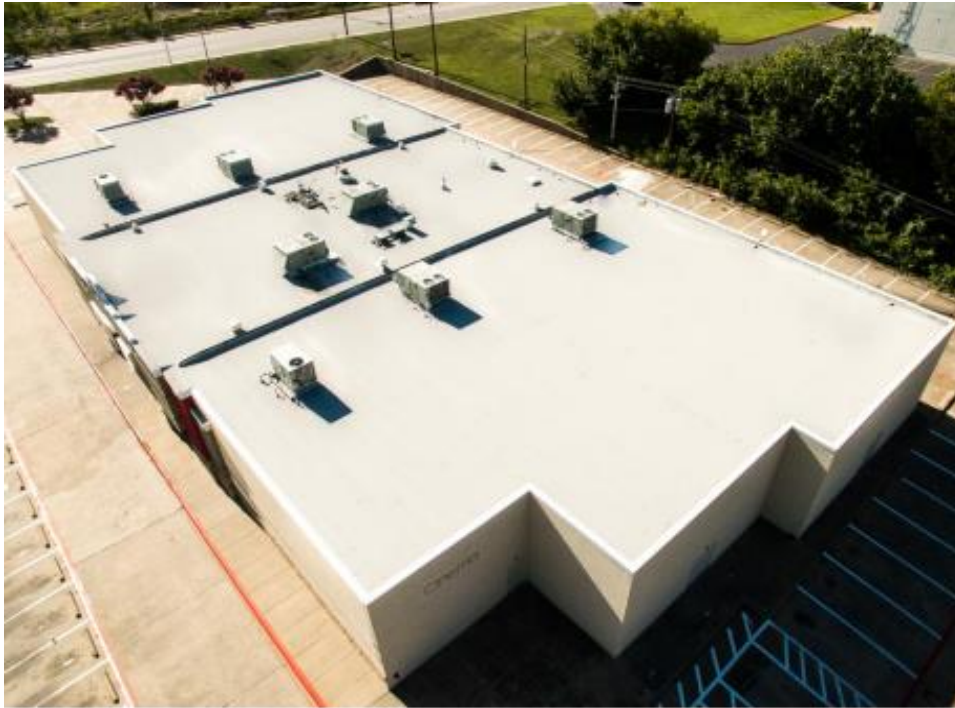
Low-slope roofing membrane installed using a propane torch and consisting of modified bitumen cap sheet and base sheet.
