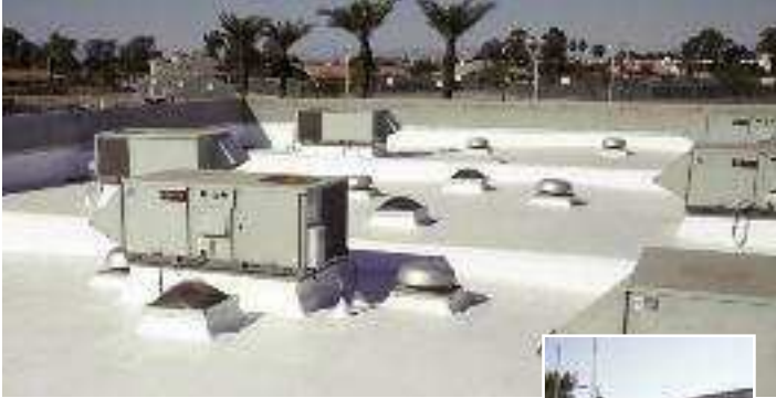
Southwest High School, El Centro, Calif. 76,000 square feet of JM PVC-60 Roofing Contractor: Roof Construction, Escondido, Calif. Owner: Central Union High School District
