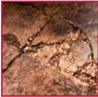
SLAB CORNER BREAKS
