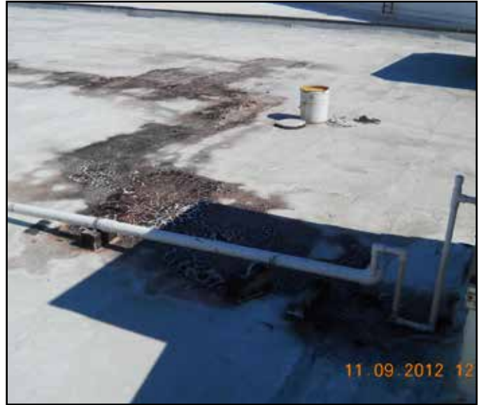
Poorly maintained condensate drain lines
