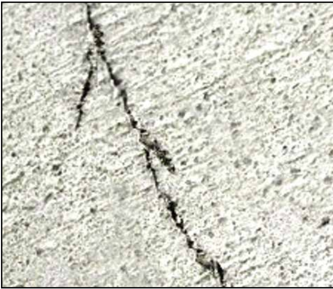
Crack before coating
