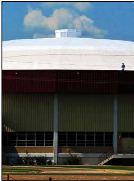
Roof with moisture contamination
