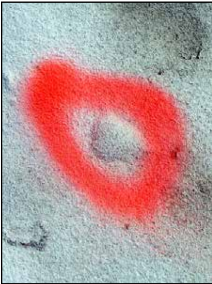
Blister due to contamination
