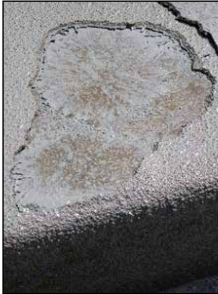
Area underneath removed blister
