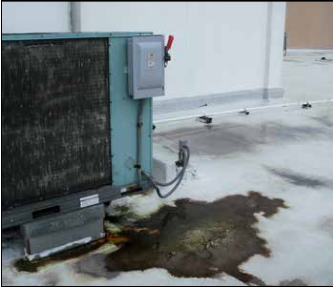
Disconnected condensate drain lines
