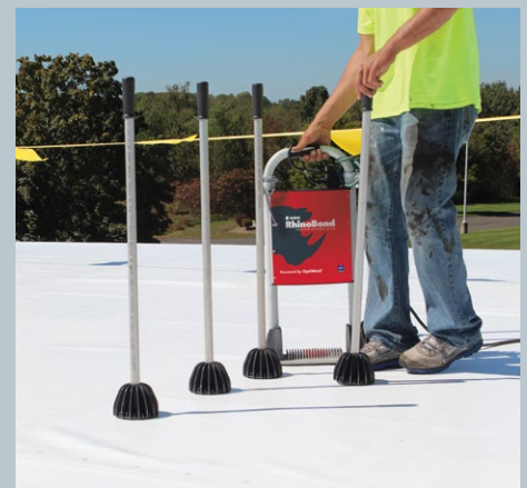
3. After the membrane is installed, weld each plate using the RhinoBond tool.
