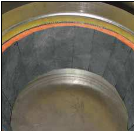
Figure 29 - View of insulation inside reducer
