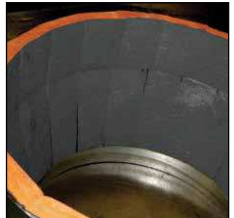
Figure 30 - View of reducer insulation to flange insulation
