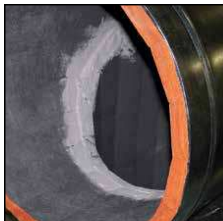
Figure 22 - Coating on the inside edge of Tee
