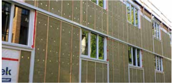
Example of insulation retained by mechanically attached impaling pins between vertical wood framing (adhesive stick-pins are not considered a long-term support strategy).
