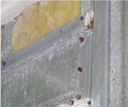
Image 1: Corrosion of the studs and fasteners on a 7-story concrete and metal framed building in a hot-humid climate, 7 years after the building was completed. The exterior water and air control layer of this building was a mechanically-fastened building wrap that was not detailed to be sufficiently airtight, nor was it sufficiently water-vapor impermeable to counteract high moisture drive from the exterior to the interior.
