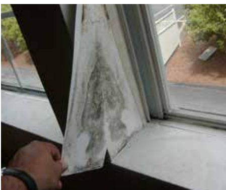
Image 3: Mold on the backside of a vinyl wall covering at a 4-story hotel. Vapor barriers such as polyethylene sheeting, foil-faced batt insulation, reflective radiant barrier foil insulation, and any impermeable wall coverings should be avoided on the interior of air-conditioned spaces in any climate, but especially hot-humid climates where buildings experience increased vapor drive from the exterior to the interior. Interior vapor barriers provide both a cold condensing surface for water vapor and restrict interior drying.
