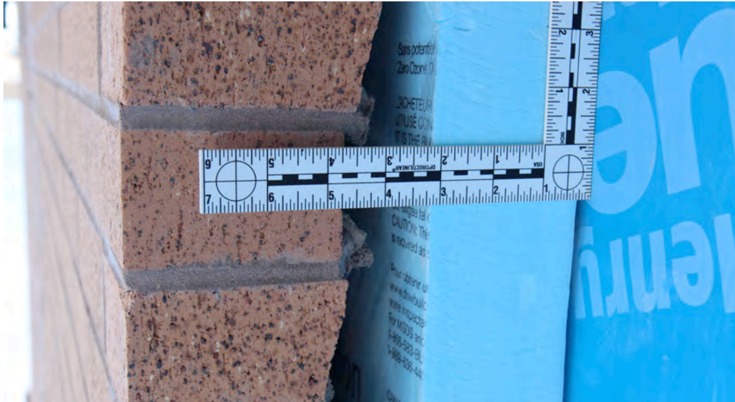
Figure 8: Actual air gap (1/4" or 6 mm) measured behind insulation on a school enclosure
