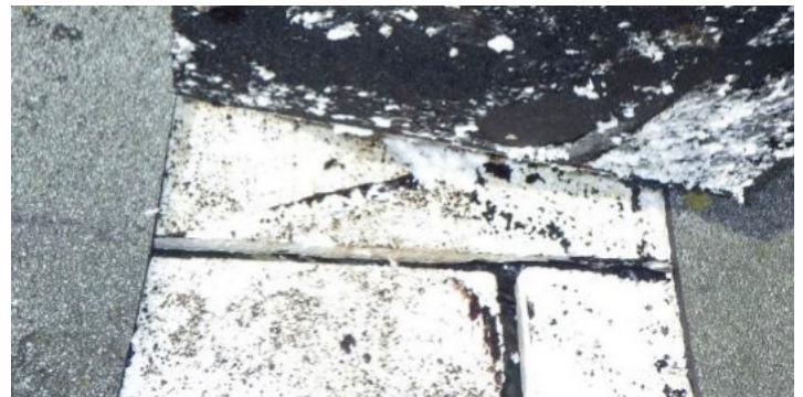
Figure 2 Permanent shrinkage of EPS insulation in a conventional roof assembly, potentially due to high in-service temperature or initial application into hot asphalt adhesive.
