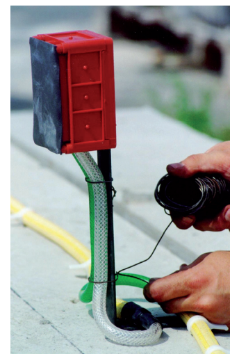
Junction boxes for easy connectivity to hoses
