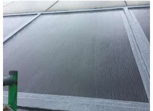
Sikalastic® Clearglaze is applied by foam roller at 20 mils WFT (80ft 2 /gal) per coat. Lap up onto the installed RoofPro membrane 2 inches butting up against the mullion.
