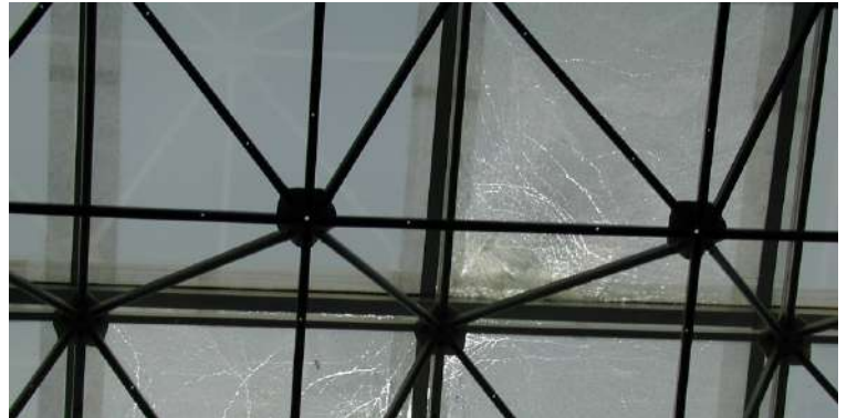
Skylight was protected with Sikalastic Clearglaze. After Hurricane Charlie, the skylights shattered but remained in place.
