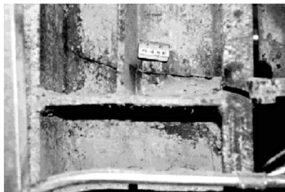
Figure D2.2 — Fracture of Welded Beam-to-Column Connection in Northridge Earthquake
