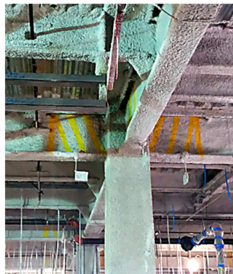
Figure D4b.3 – Protected Zone Marking for an RBS Connection in the Field (Sprayed on Top of Fireproofing)
