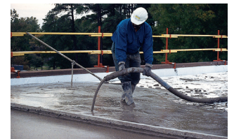
A top layer of insulating concrete is placed over the Insulperm, filling the holes in the Insulperm and locking it into the system without the use of fasteners.
