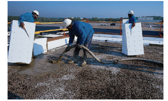
Decreasing thicknesses of Insulperm Insulation Board form the slope-to-drain contour of the finished system.
