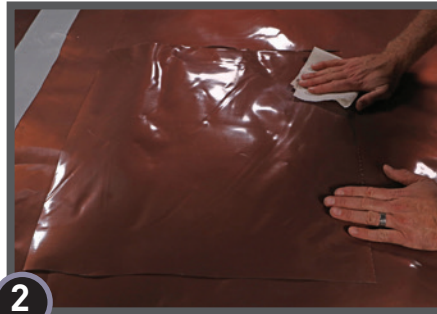
2 Measure and cut a piece of Drago Wrap to cover damaged area 6" in all directions. Clean area of adhesion.
