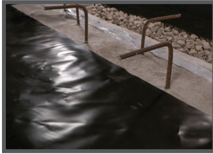
Onto Interior Grade Beams at Impediments: Seal Pango Wrap to concrete with Pango Bond and Pango Term Bar.
