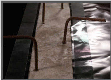
At Interior Grade Beam Impediments: Install Pango Claw onto the terminating edge of Pango Wrap.
