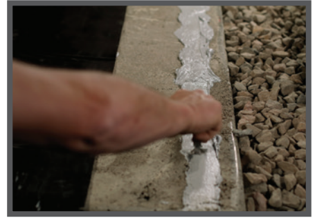
At a Location Designated by the Design Team: Seal Pango Wrap to concrete with Pango Bond and Pango Term Bar.
