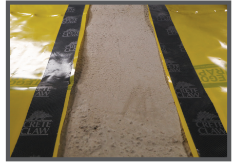
At a Location Designated by the Design Team: Install Stego Crete Claw onto the terminating edge of Stego Wrap.
