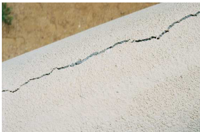
Photo 1: the large crack in the parapet requires elastomeric crack filler, followed by waterproofing with glass fiber mesh installed around the parapet and a minimum of 6" down each side.
