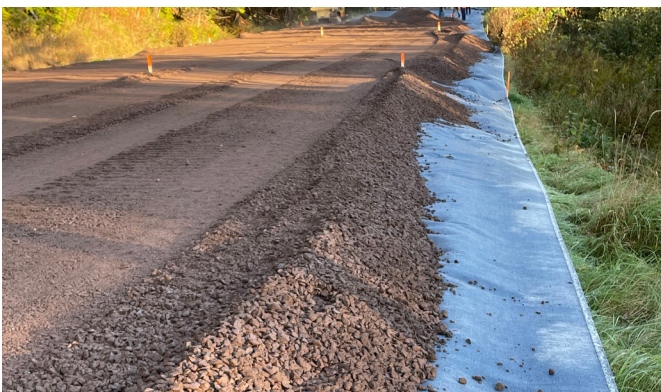
Image 8: Edge termination on side of embankment into ditch line (right side)
