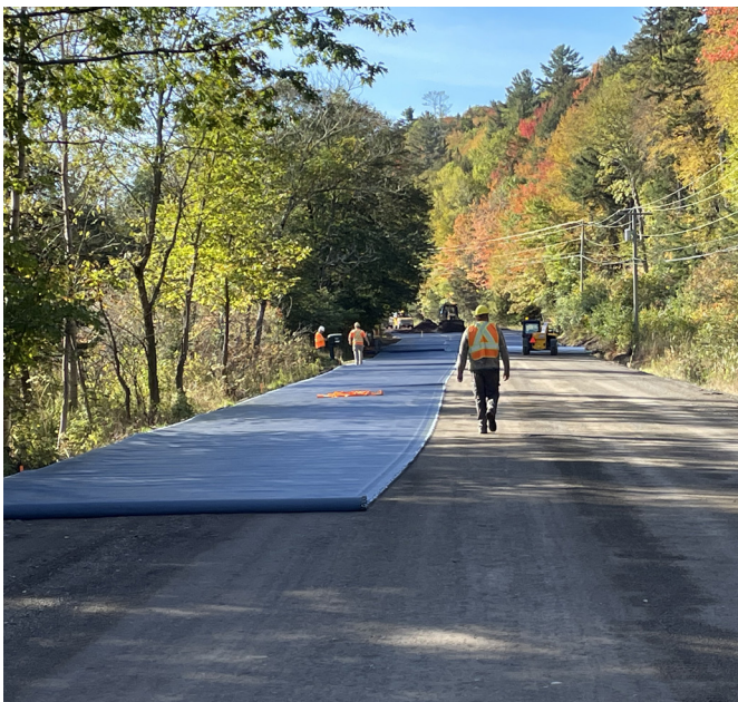
Image 1: MIRAFI H 2 Ri installed parallel to planned traffic flow over a prepared subgrade
