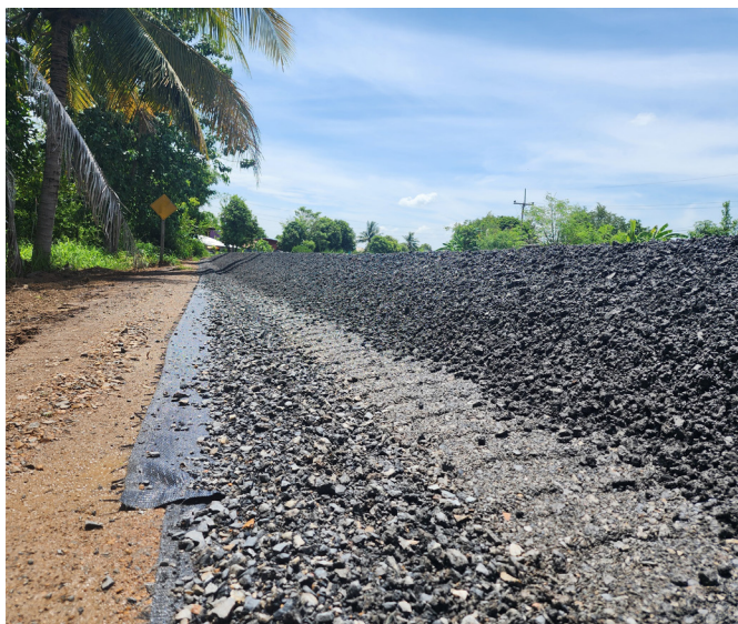
Image 9: Daylighting installation using Rip Rap to cover the exposed edge of MIRAFI H 2 Ri
