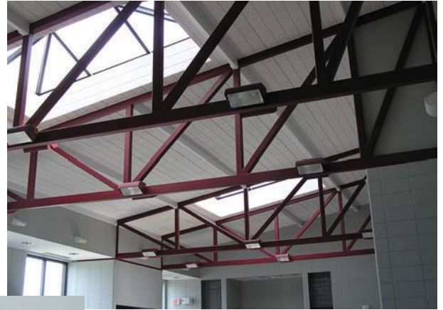
Carlisle County High School Bardwell, KY Tectum V-Line Ceiling Panels
