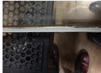
Sealant blow by
