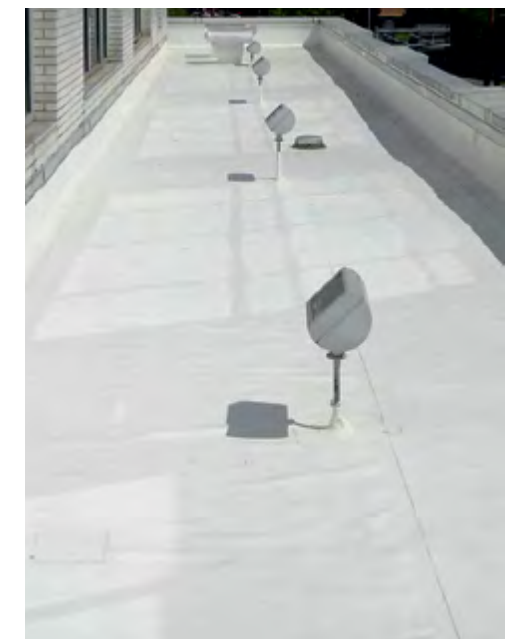
White single ply roof, cleaned and ready to be coated with AlphaGuard.
