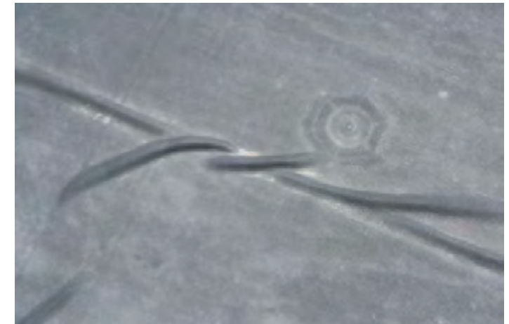
Wrinkles in EPDM will telegraph through the AlphaGuard system. It is necessary to make these repairs before applying AlphaGuard.
