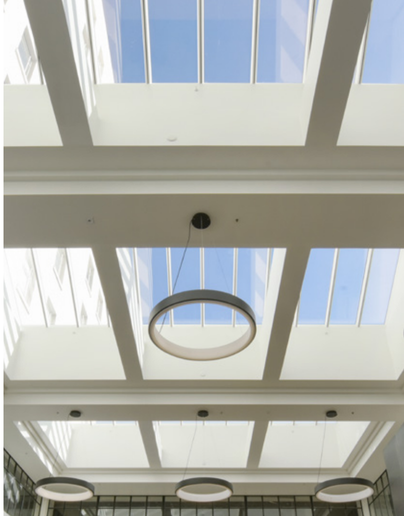
VMS Ridgelight, The Leamington Hotel, Oakland, CA
