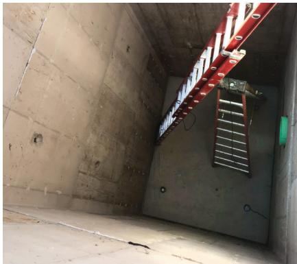
Roaring Fork Club, Colorado, USA Lift Station • Xypex Bio-San C500
