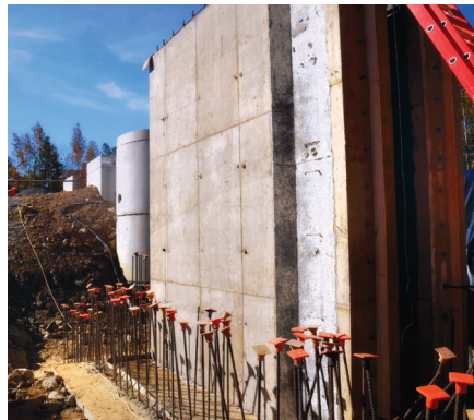
Chatham Park WWTP, North Carolina, USA Catch Basin & Manholes • Xypex Bio-San C500
